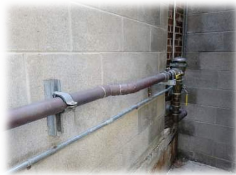
Second backflow preventer in garage space
