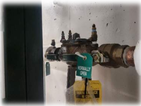
Reduced pressure backflow preventer at tap
